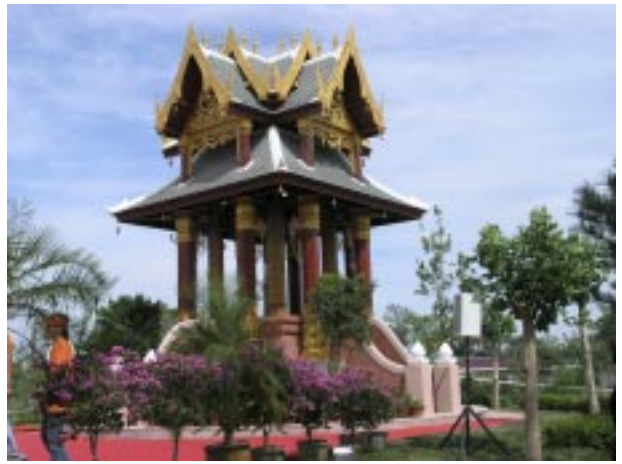
At left: The Thai Pavilion under construction in China; above: the gift fit for a king, delivered by Trans-Link Relocation to China.
