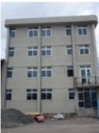
Packtra's new head office under construction. The company is also building a new bonded warehouse.
