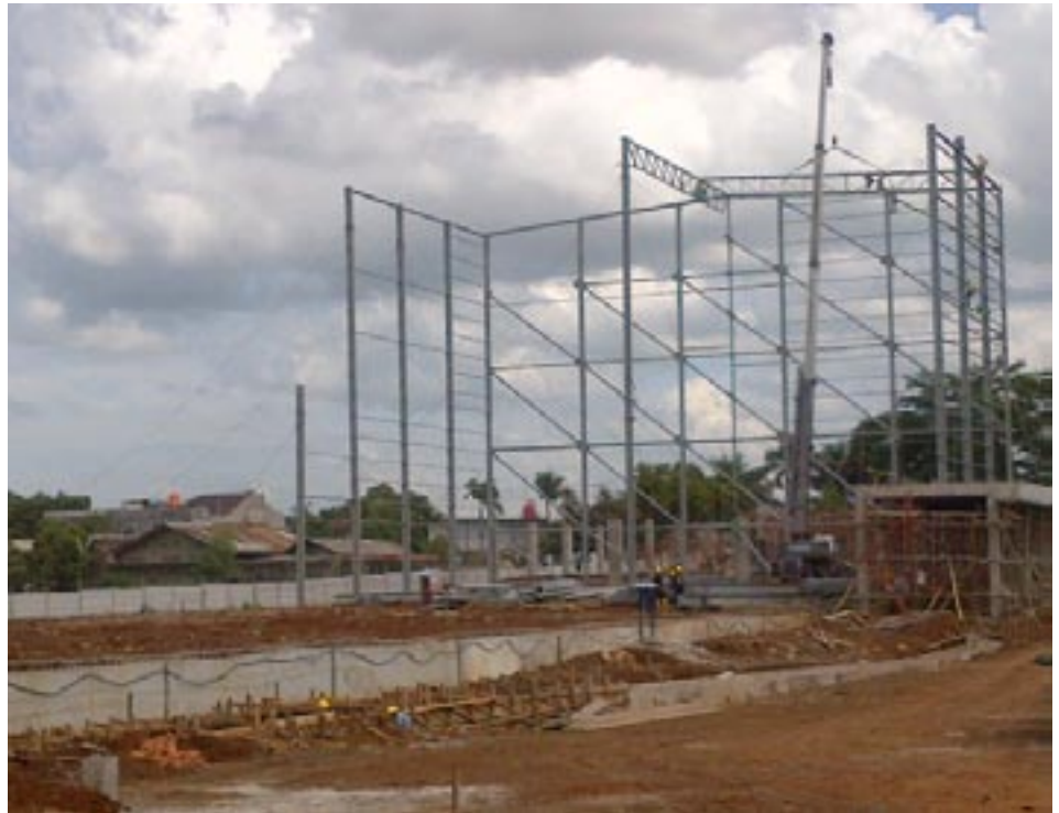
A skeleton of the building is erected on the new lot purchased by Santa Fe Jakarta.
